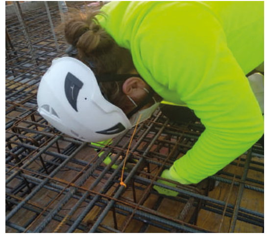
Operario instalando sensor CoSMoS™
